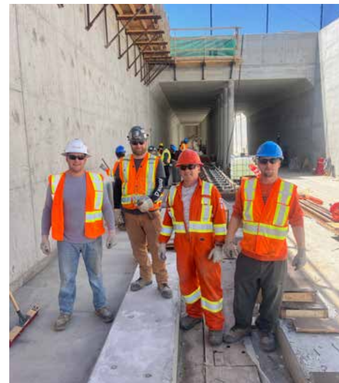
Members Mikael Lalama, Brandon Hockley, Rocky Lalama, and Alex Lalama installing railroad jigs on a large rail project in Ottawa for PNR RailWorks
