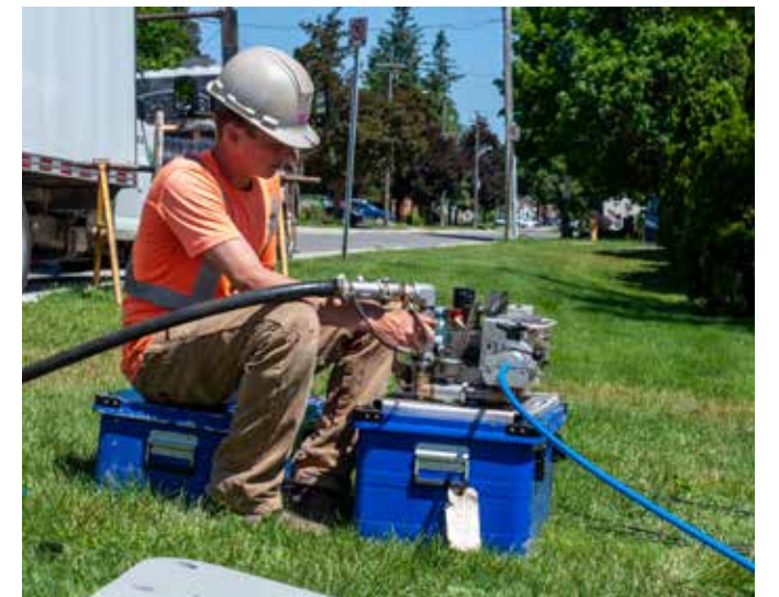
Travis Copeland, a former Local 1059 apprentice now with Pickard Construction, is fibre jetting on Tenth Street and Second Avenue in Owen Sound.
