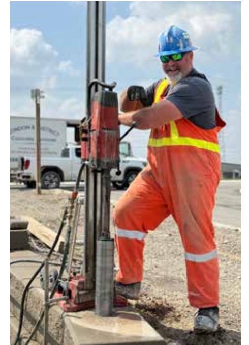
Member Joe Swain of London District Cutting and Coring working on a retaining wall fence
