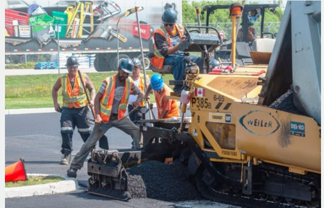
Members from Del-Ko Paving & Construction and K & H Asphalt, Sealing & Striping re-paving The Local 1059 parking lot
