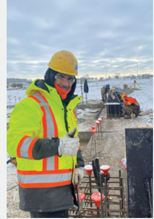
Apprentice Mario Carvalho of EllisDon at the in-progress battery plant for GM CAMI in Ingersoll
