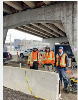
Freddy Ford, Kale Brooks, Scott Lennox of Weathertech Restoration Services repairing the Adelaide St. bridge
